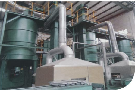
Mixing system Workshop
